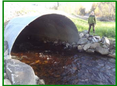
Above: TTCD Board Chair Ron Stanek with newly installed Tyonek Creek culvert.
