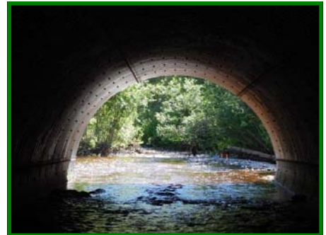
Above: Partially completed culvert installation on Tyonek Creek. Photo by Dowl HKM.
